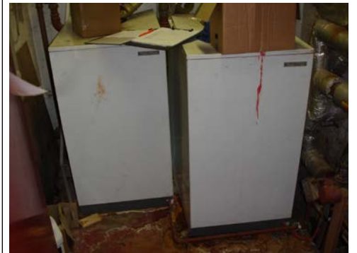
Two oil-fired Worcester boilers fitted with another MTC40
