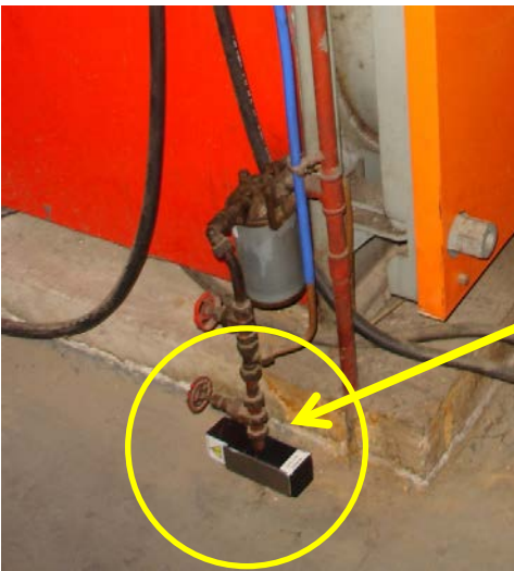
Two oil-fired Hoval SRPlus boilers, fitted with the MTC40.
